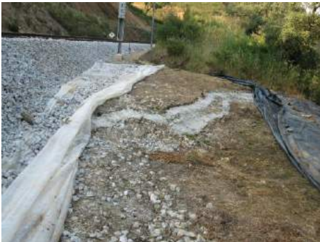
Photo 1. Instability of the embankment slope close to the railway (2011)
