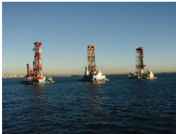
Figure 3. DM vessels in operation (by courtesy of the Tokyo/Haneda International Airport Construction Office).
