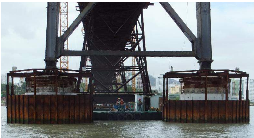
Figure 3. Metal cofferdam shall during the reinforcement foundations of one of the main towers over the sea
