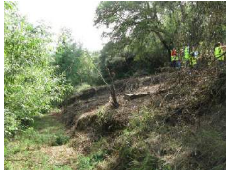
Photo 2. Instability in the embankment base slope (2011)
