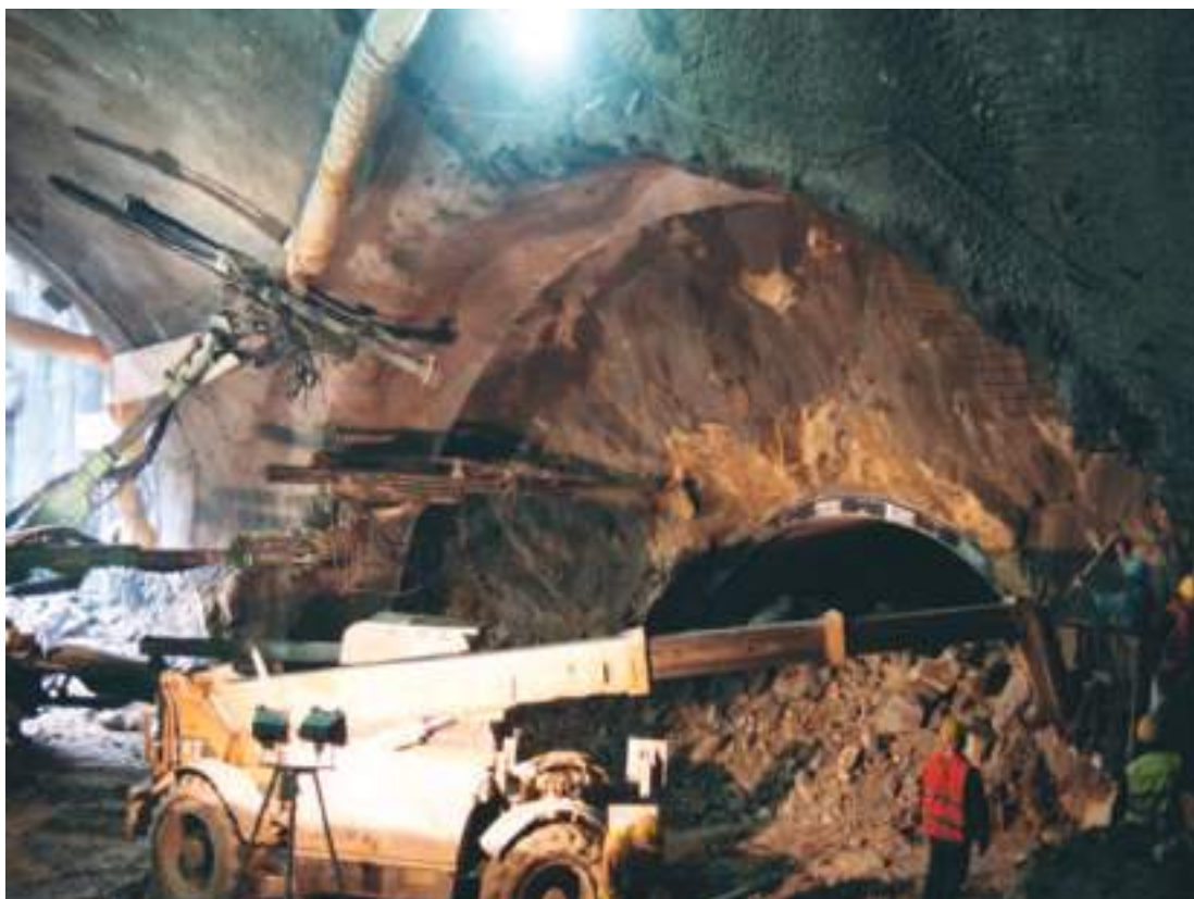
Fig. 02 Início da escavação da Caverna principal a partir da Galeria Transversal da Estação de Combatentes. Note-se a presença das aduelas do túnel de via anteriormente executado com TBM. Beginning of the excavation of the main cavern from the transversal gallery of Combatentes Station. The segments of the rail tunnel previously constructed by TBM can be seen at the excavation face.
