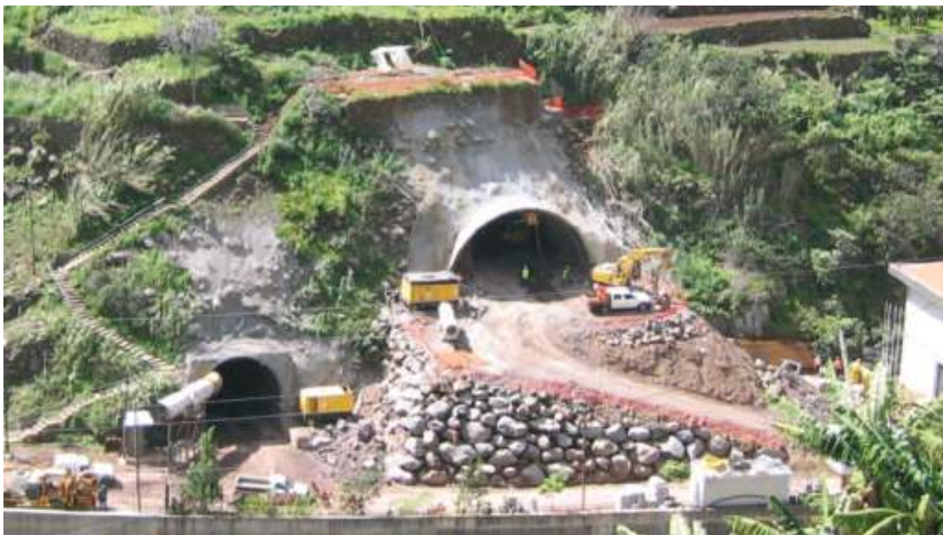
Fig. 05 Emboquilhamentos da galeria e do túnel auxiliar. Portal of the gallery and of the secondary tunnel.
