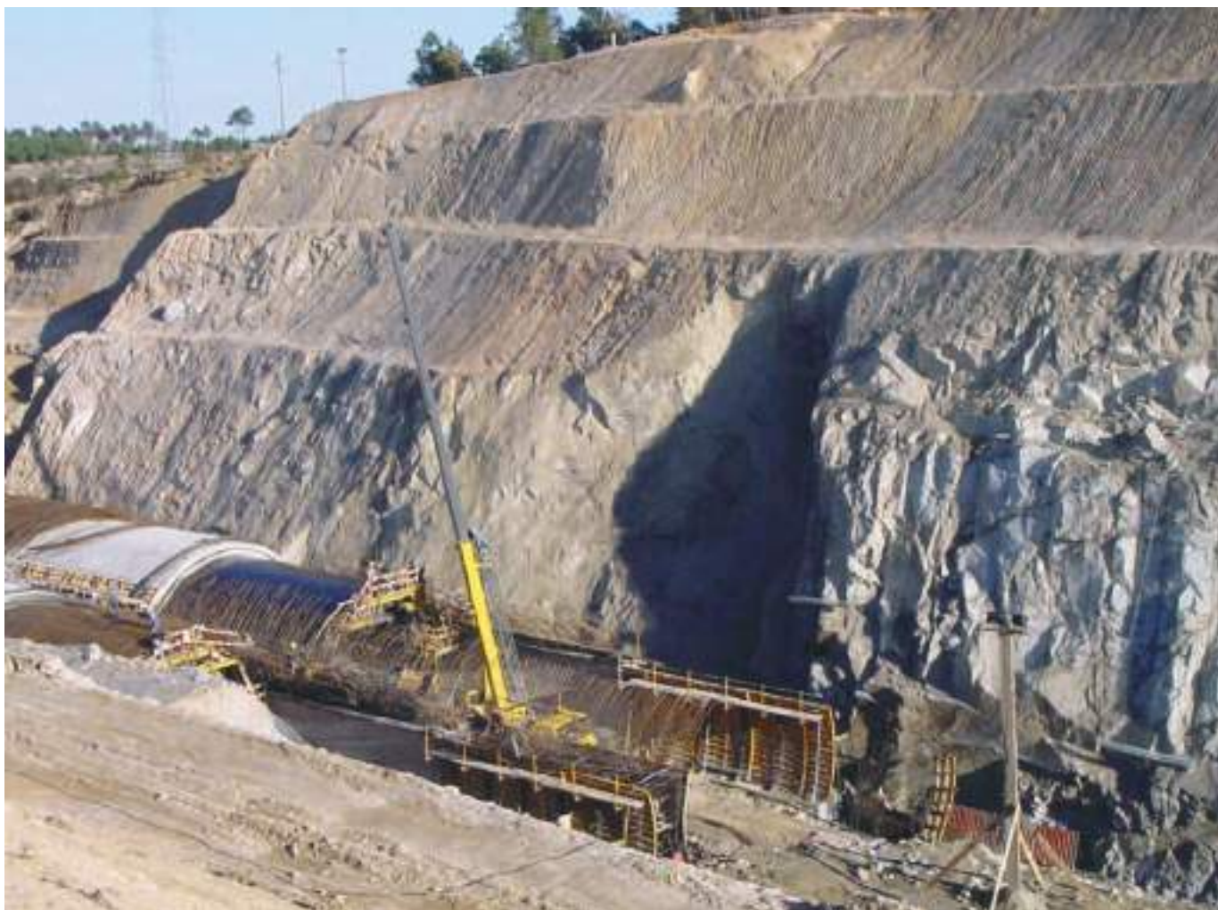
Fig. 05 – Túnel do Barracão - Cunha resultante do deslizamento de material rochoso no talude Nascente, com cerca de 400 m 3 e aspeto geral dos trabalhos. Barracão Tunnel – Wedge resulting from landslide of rocky material in the eastern embankment, with approximately 400 m 3 and general aspect of the works.
