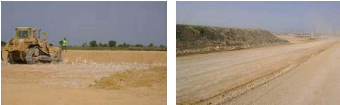
Figure 5. PLLN general platform with query debris and preloading embankment, with clayed soils
