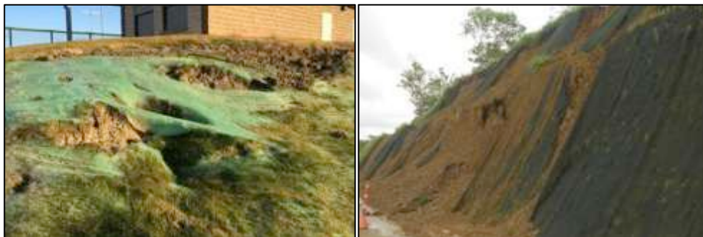
Figure 1. Surficial slope instability incorrectly repaired with turf reinforcement mats
