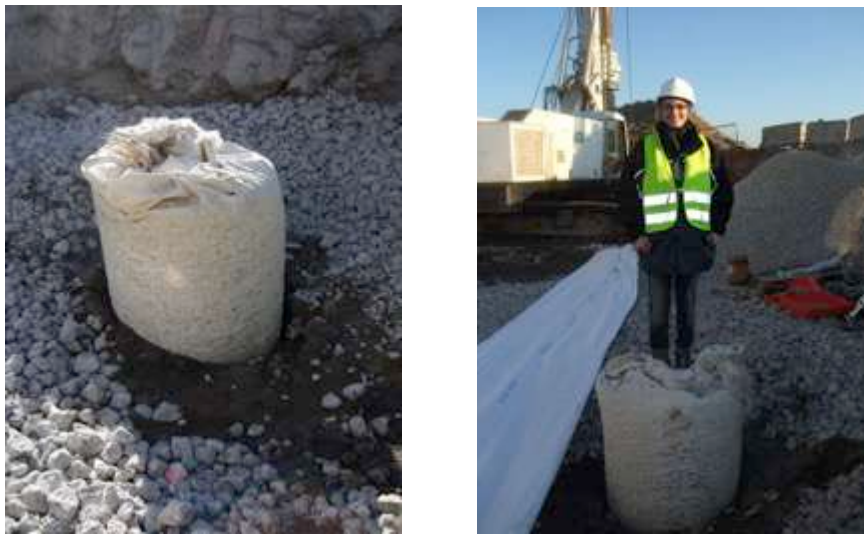
Figure 3. Demonstration of the confining capability of high strength geotextile encasement for GEC “in air”
