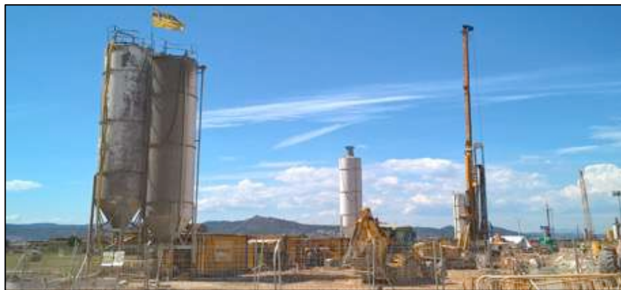
Photo 1 and 2. Keller equipment for jet grouting with the must of aprox. 35 m.
