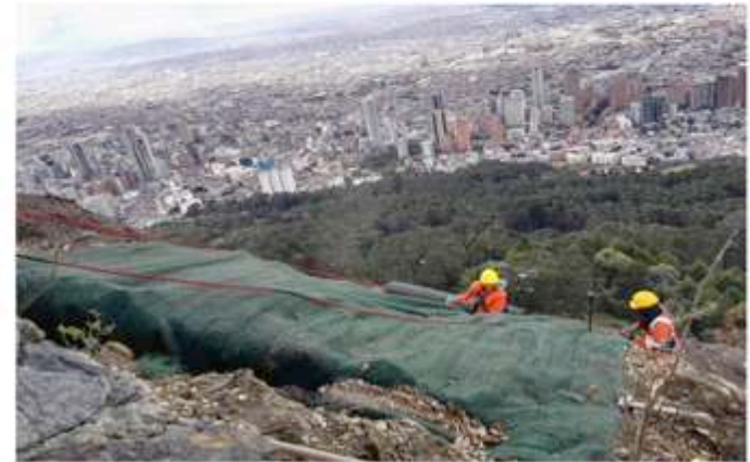
Slope Protection, Bogota, Columbia
